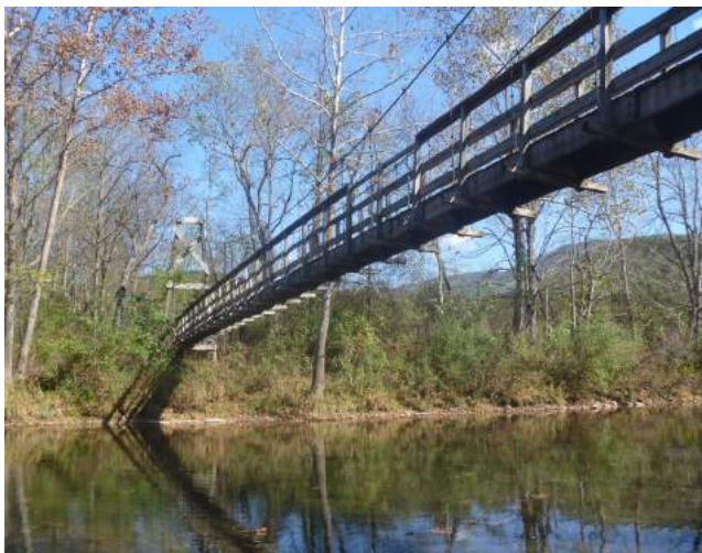
USFS GWNF North River Ranger District, Wallace Tract Swinging Bridge Demonstrating Classic Wooden Bridge Towers, Deck and Rails Photo Courtesy of C. Nelson Hoy
