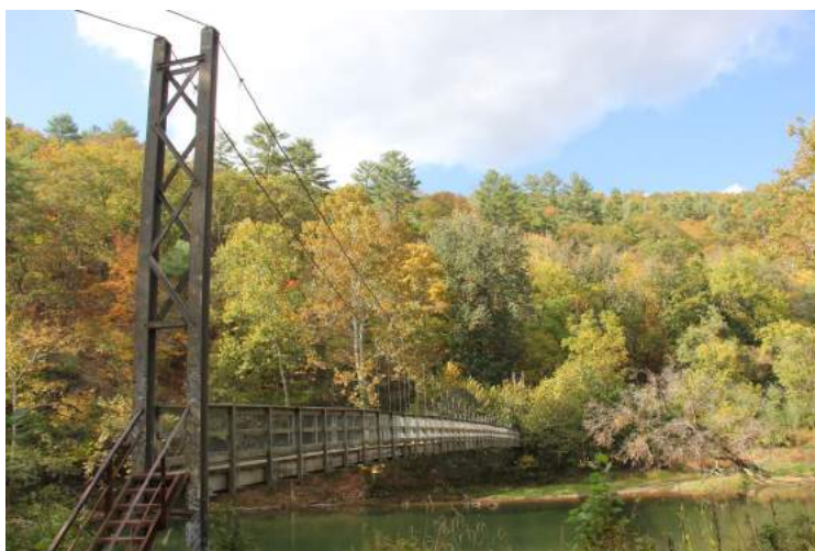
USFS GWNF Warm Springs Ranger District, Walton Tract Swinging Bridge Photo Courtesy of Kathy Farmer
