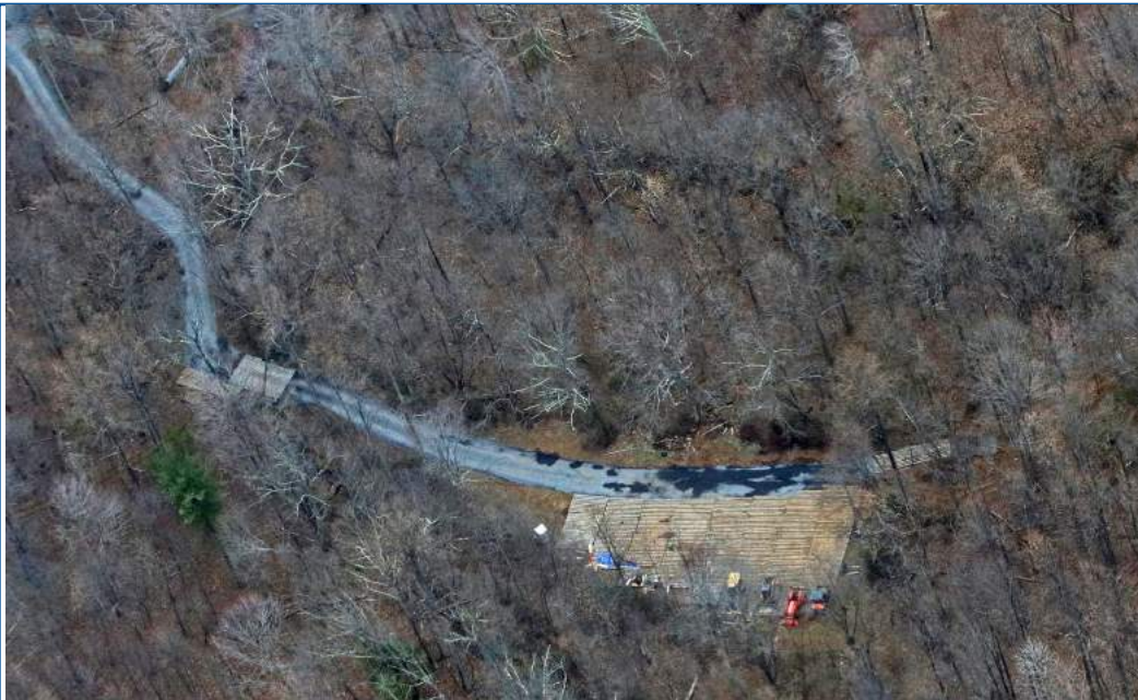
Apparent equipment staging area and new or reconstructed road and bridges observed during Pipeline Air Force surveillance flights.
